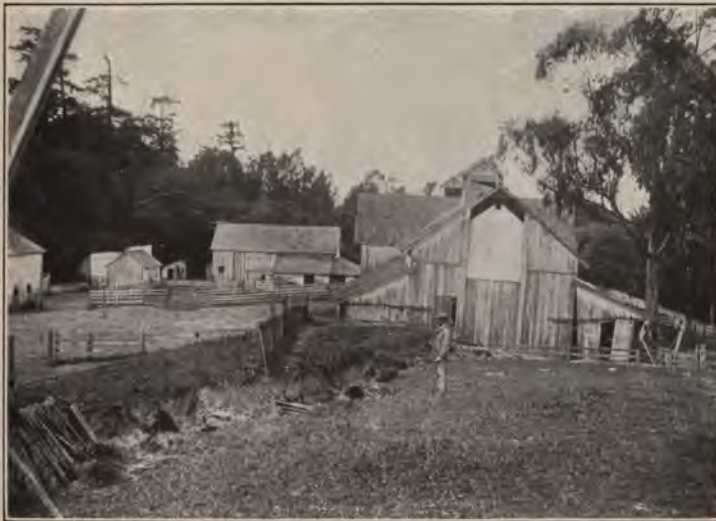
B. Barn which was tilted over a fault and dragged about ten feet.
